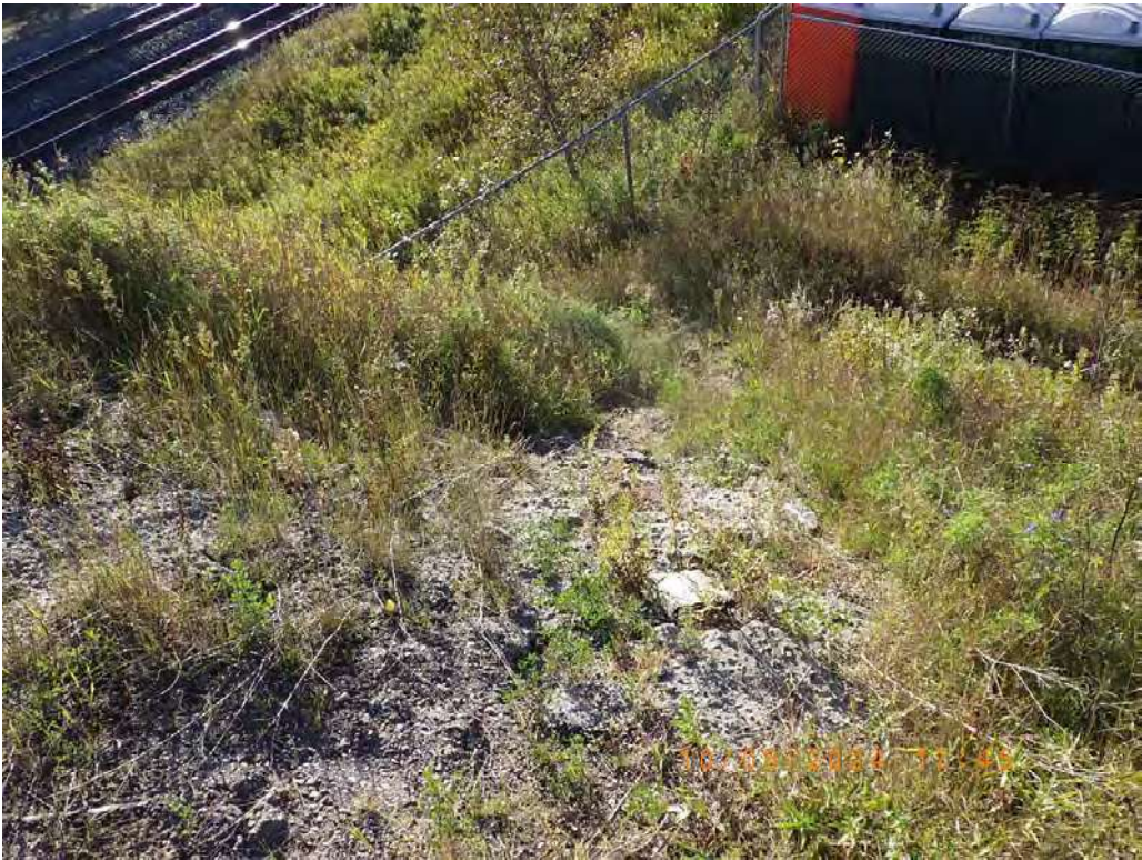
Photo 37: Erosion at embankment northwest corner of bridge.
