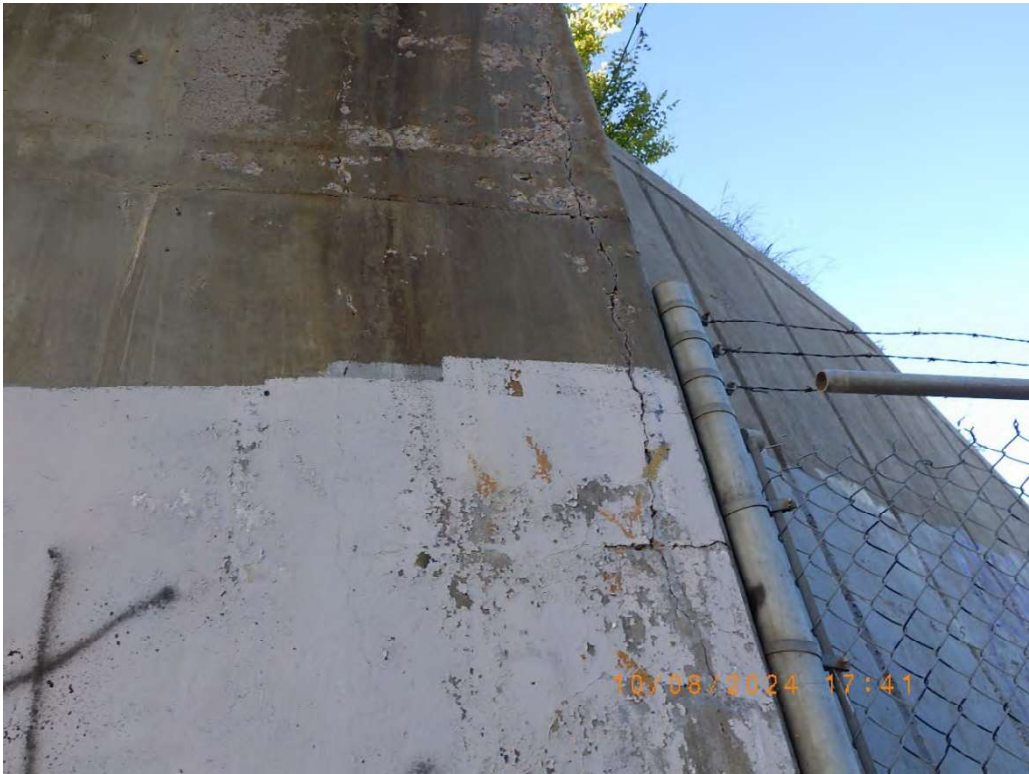
Photo 35: Vertical crack at north abutment.
