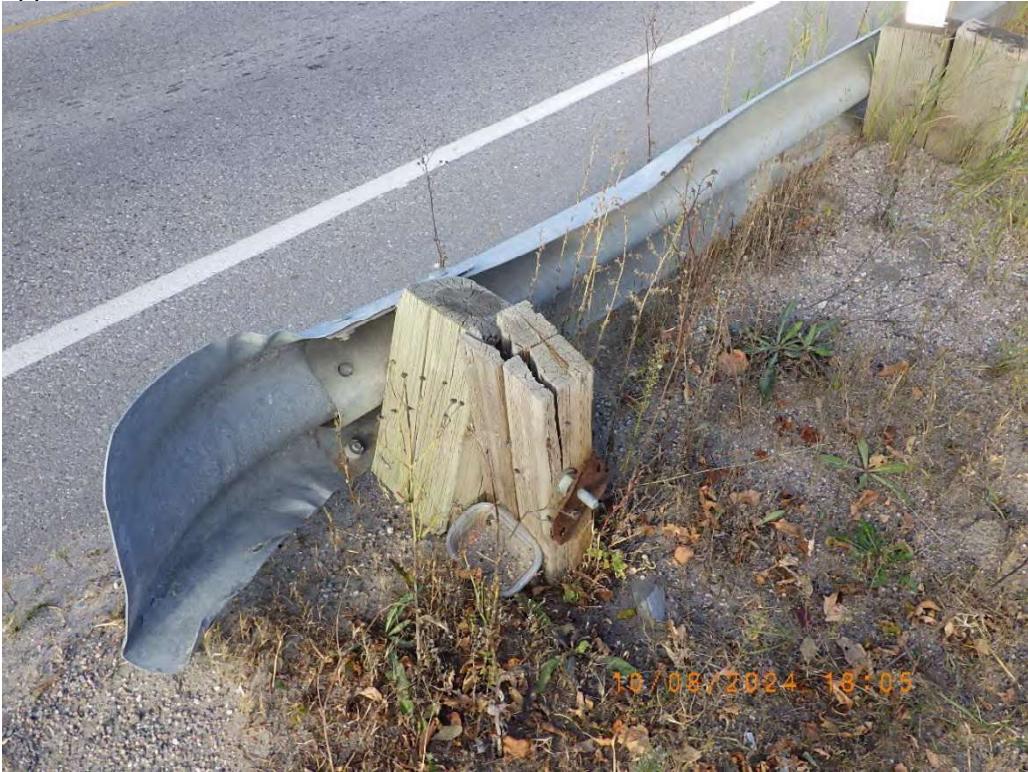
Photo 42: Rotated offset timber at southeast corner of site (typ.).
