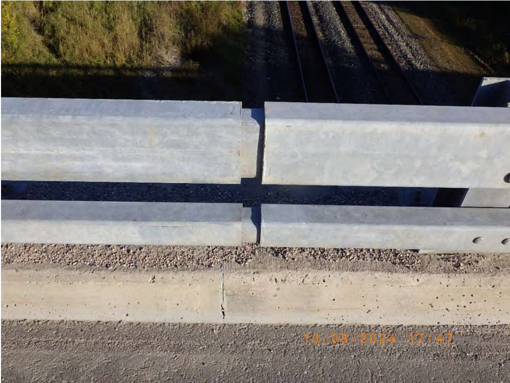
Photo 33: Wide gap at steel beam splice.
