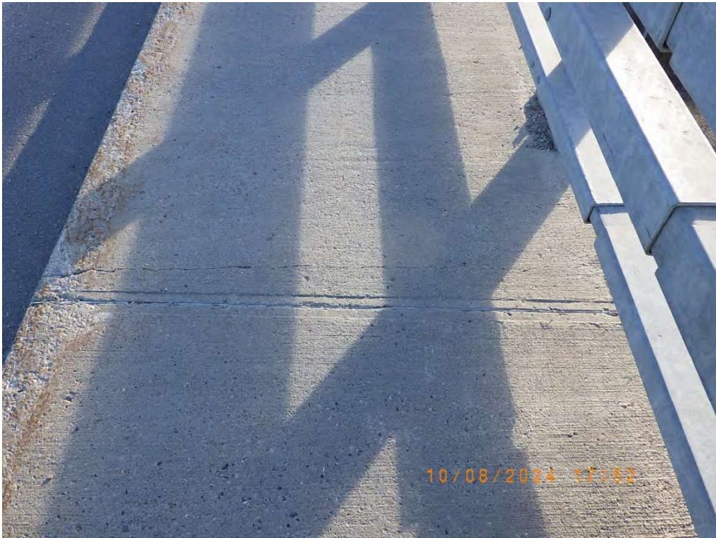
Photo 30: Medium transverse crack in sidewalk.
