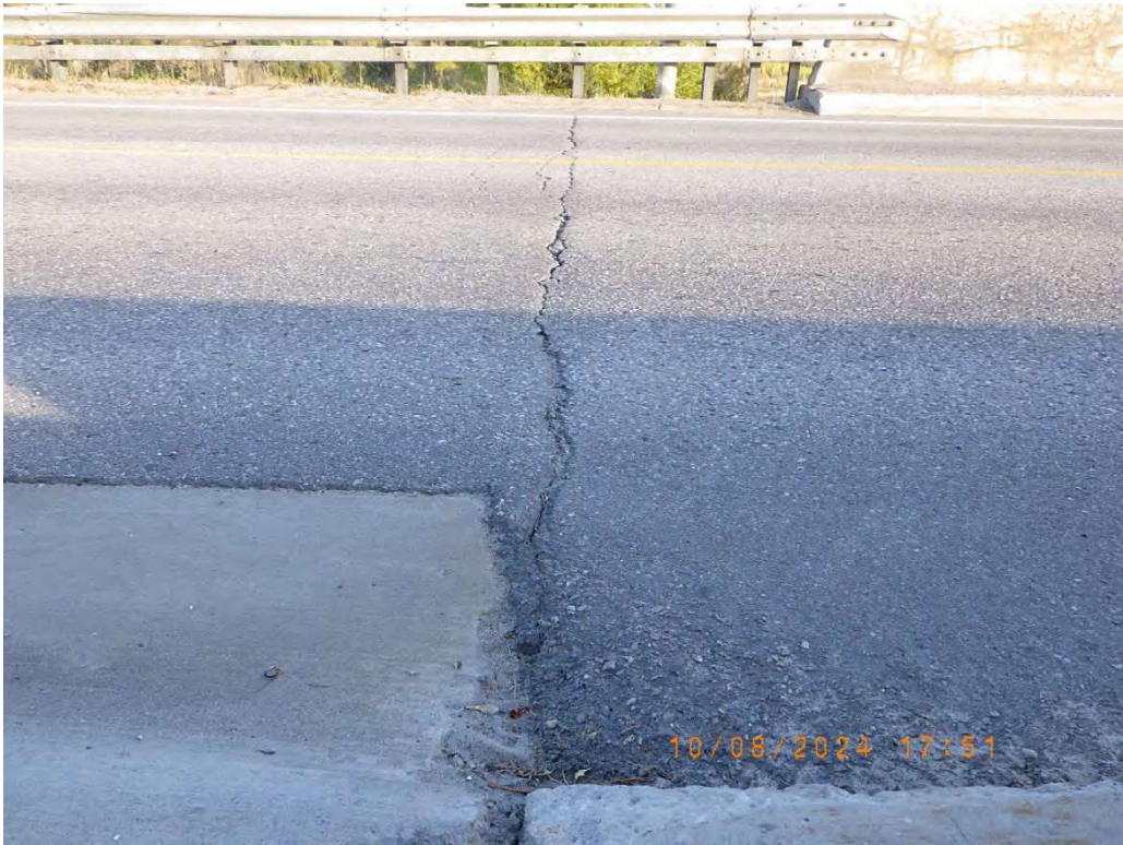
Photo 21: North approach slab joint.
