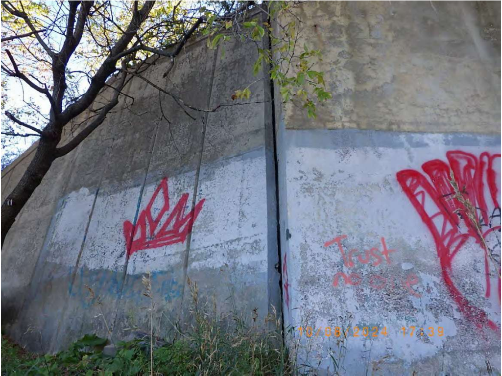
Photo 34: Wide gap between southeast wingwall and south abutment (typ.).
