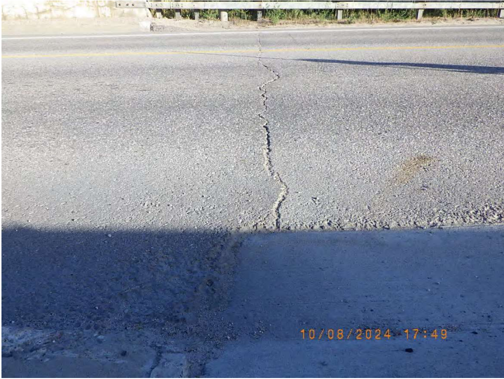
Photo 22: South approach slab joint.
