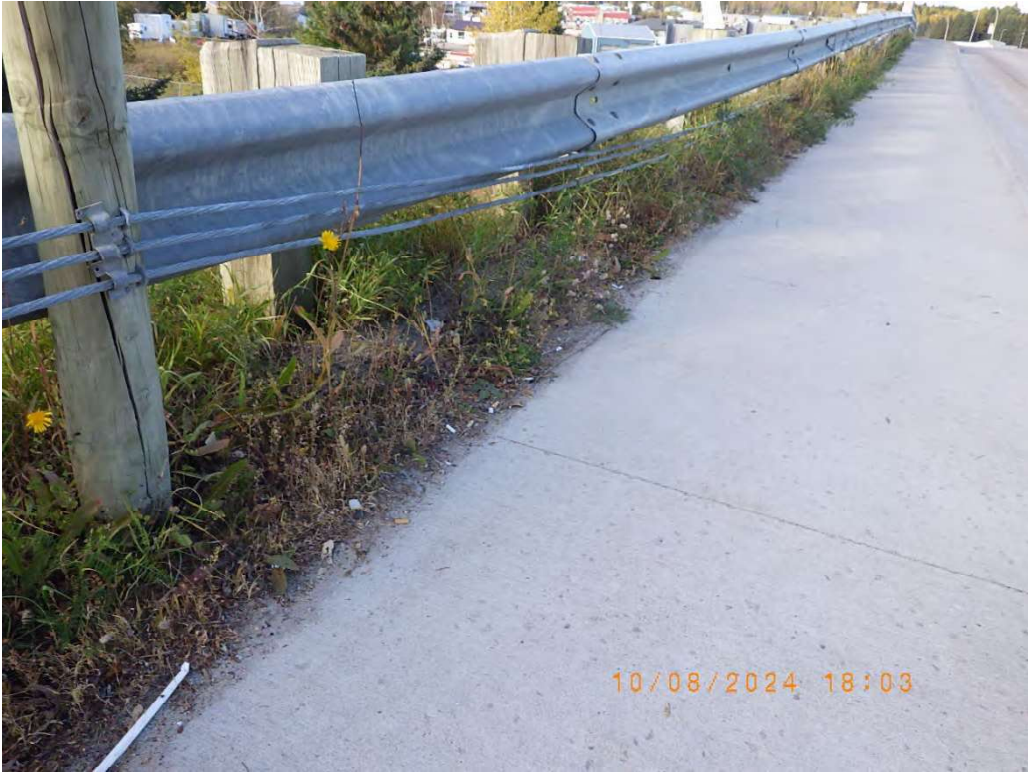
Photo 40: Loose cables at south approach.
