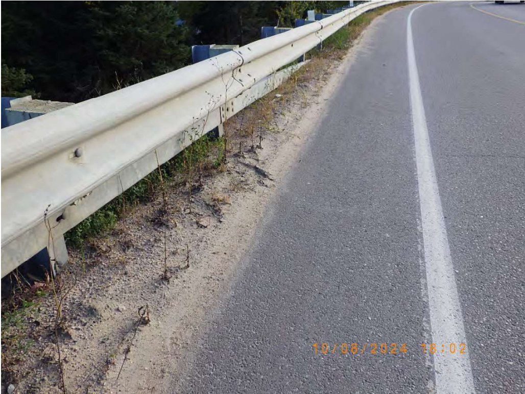
Photo 41: Gravel accumulation in front of guide rail at east side of south approach.
