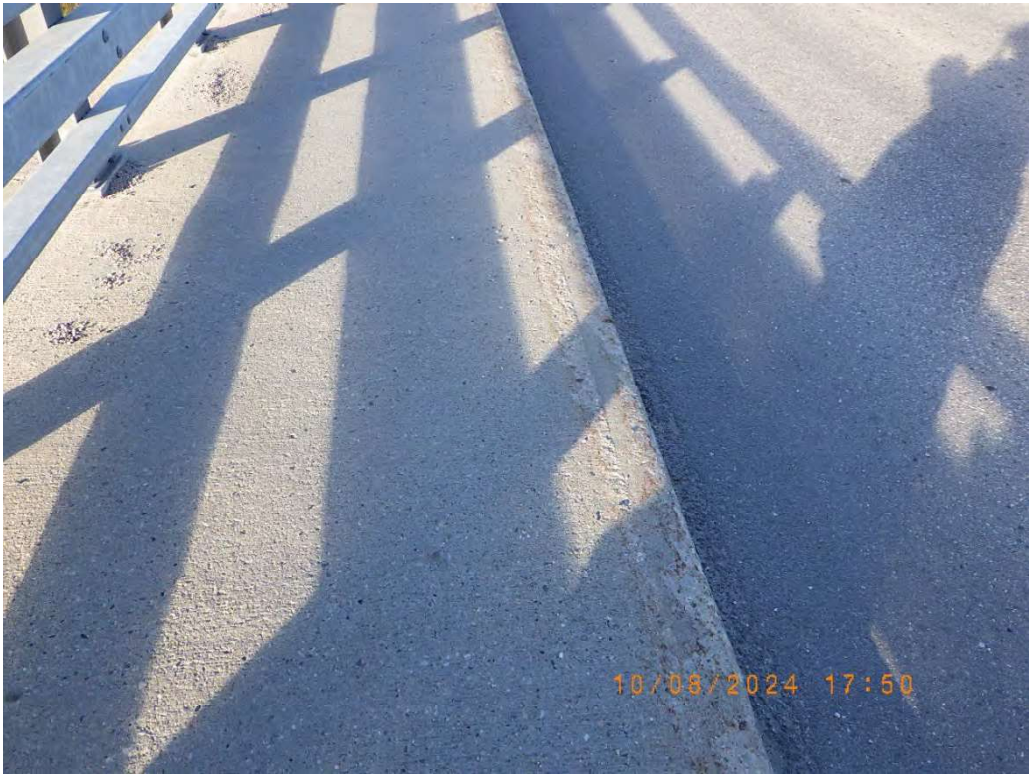
Photo 29: Abrasion damage along face and top edge of sidewalk.
