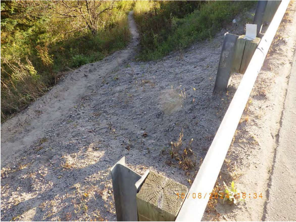
Photo 38: Erosion at embankment southeast area of site.
