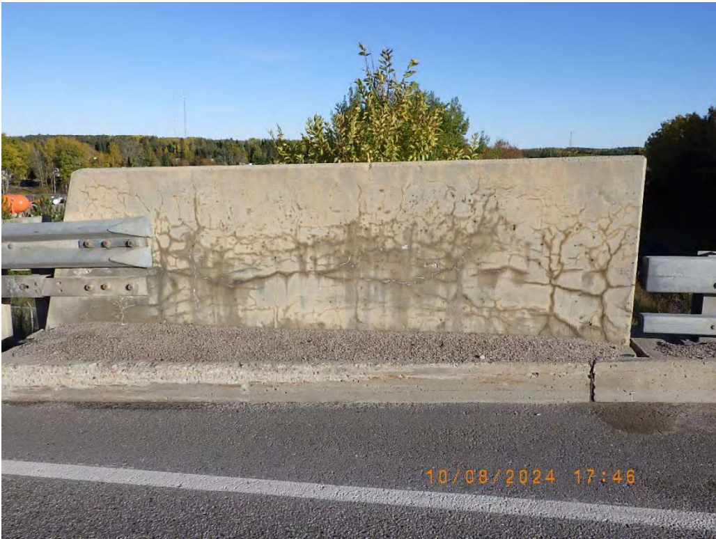
Photo 32: Scaling, delamination and cracks at northeast parapet wall (typ.).
