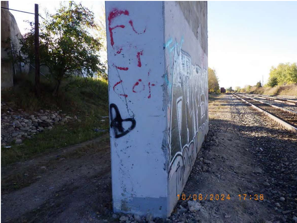
Photo 36: Corner spalls at south pier.
