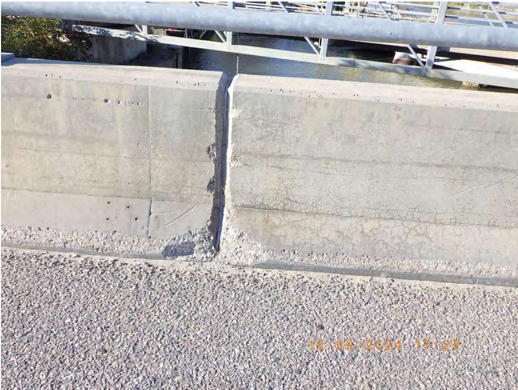
Photo 21: Spalled concrete and missing sealant at barrier joint (typ.).
