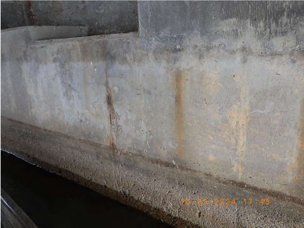
Photo 25: Narrow vertical crack at east abutment.
