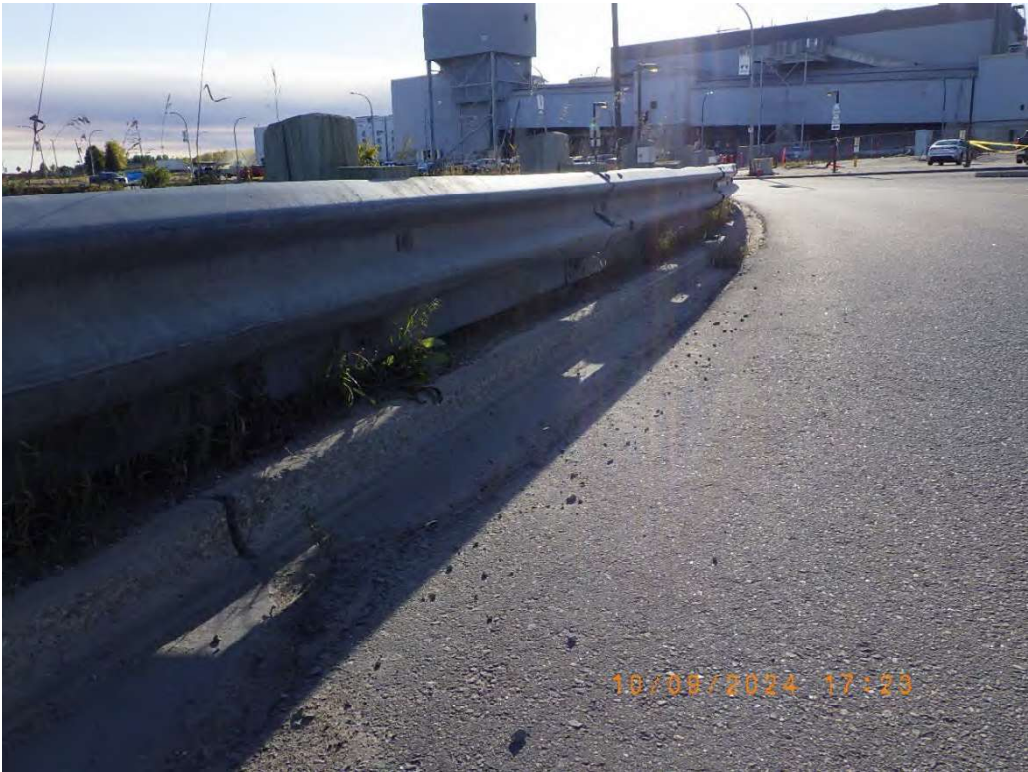
Photo 28: Abrasion damage to curb and gutter at southwest corner of site.
