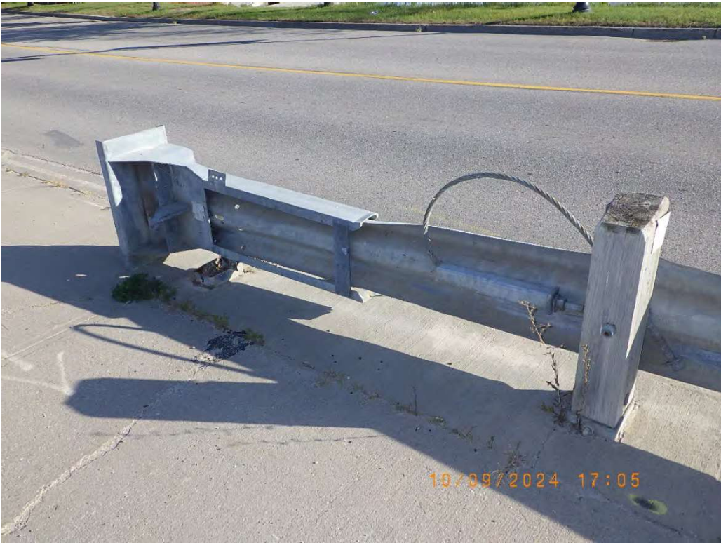
Photo 17: Broken end post (typ. 3 locations).
