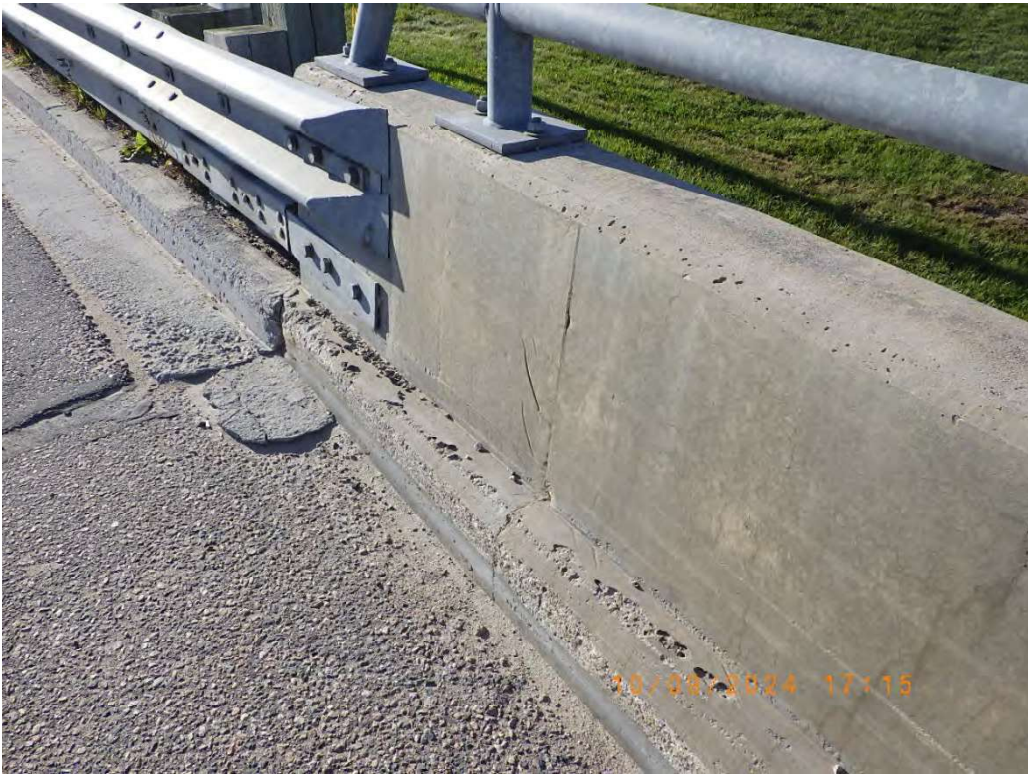
Photo 20: Abrasion damage to barriers and asphalt along side of deck (typ.).
