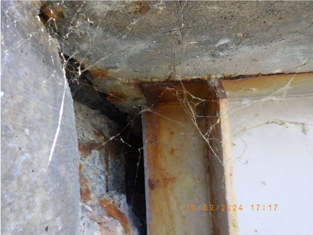
Photo 27: Spalled ballast wall at southwest corner of bridge (typ.).
