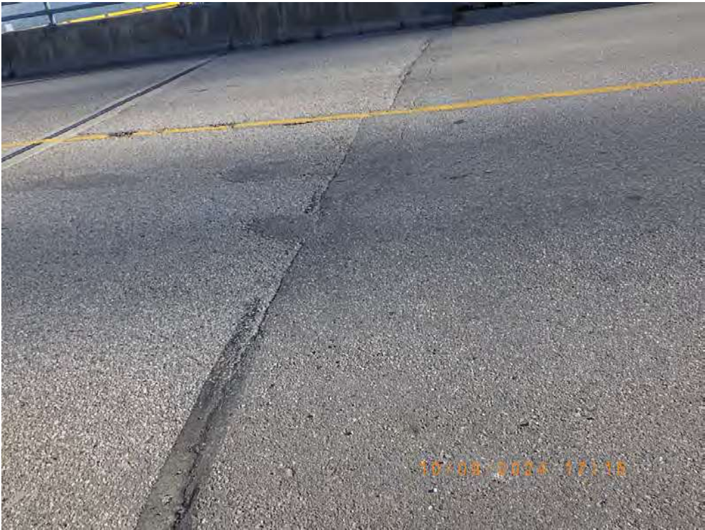
Photo 22: Poor sealant and asphalt along east approach slab joint (typ.).
