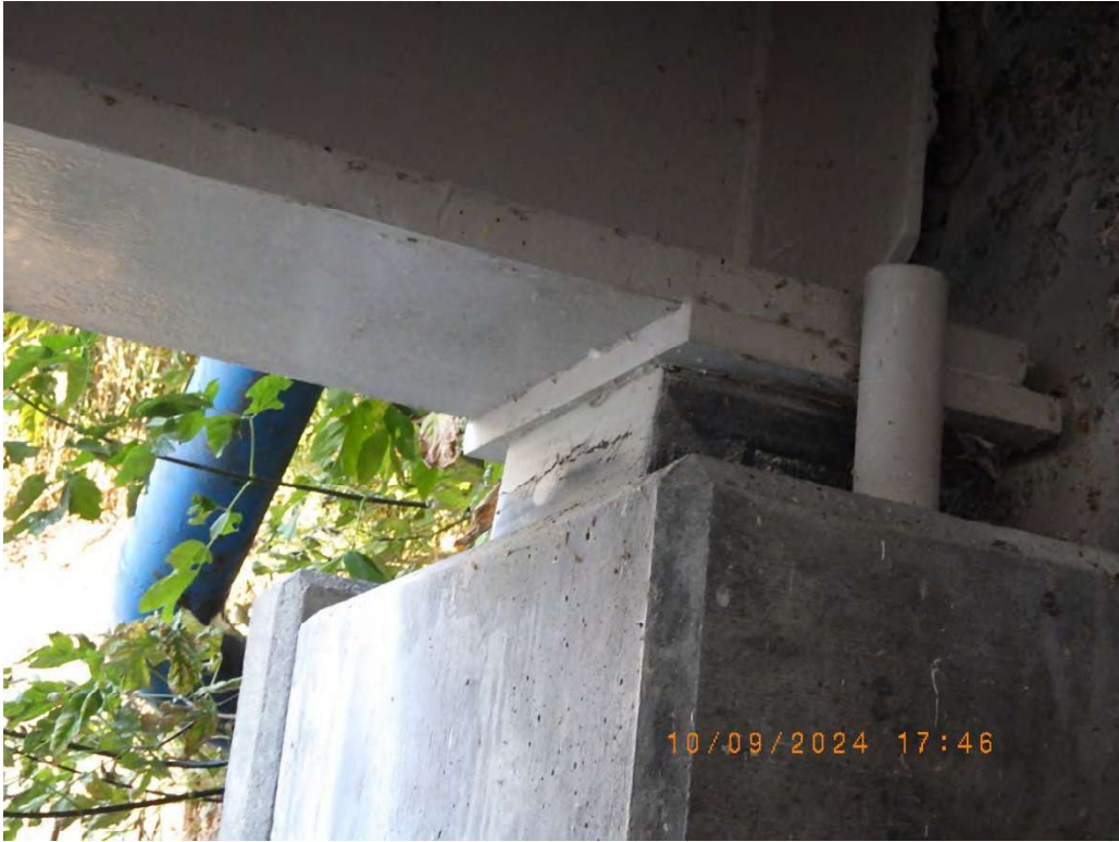
Photo 24: Bearing with horizontal cracks (typ.).
