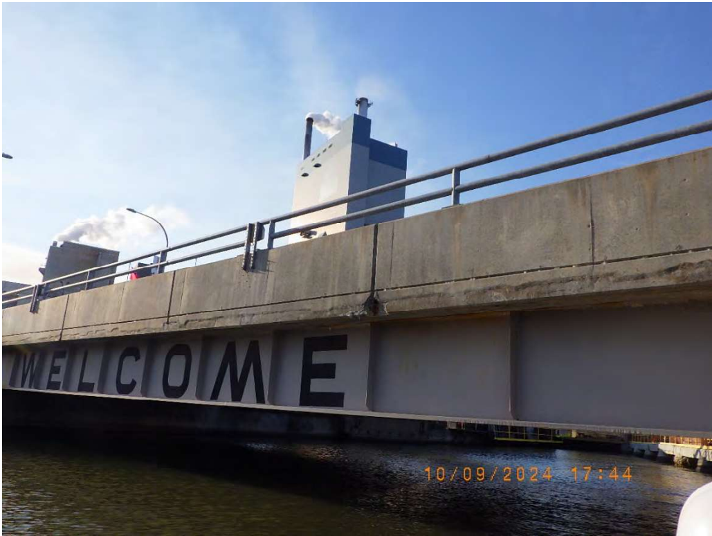
Photo 23: Spall at south face of deck.
