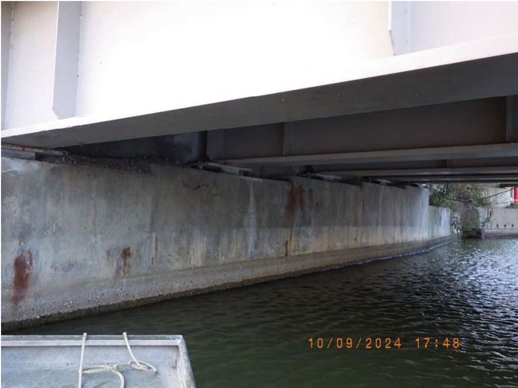
Photo 26: Delaminated concrete at west abutment.
