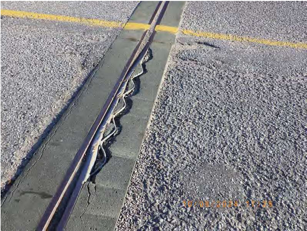
Photo 19: Abrasion damage to asphalt on deck.
