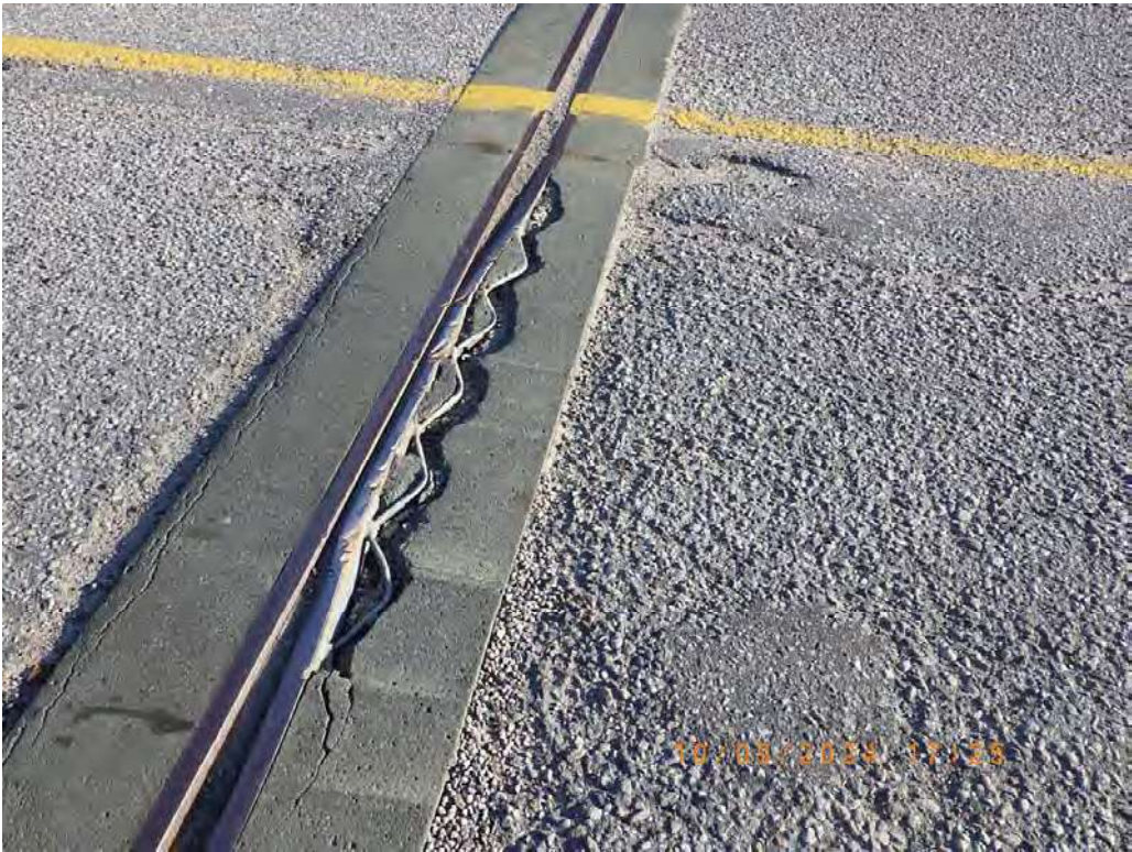
Photo 18: Deteriorated concrete at end dams, corroded armoring, broken expansion joint, and gravel accumulation above seal at expansion joint (typ.).
